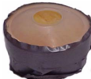
Improper cartridge filter combination. (Duct tape holding two different brands together)
